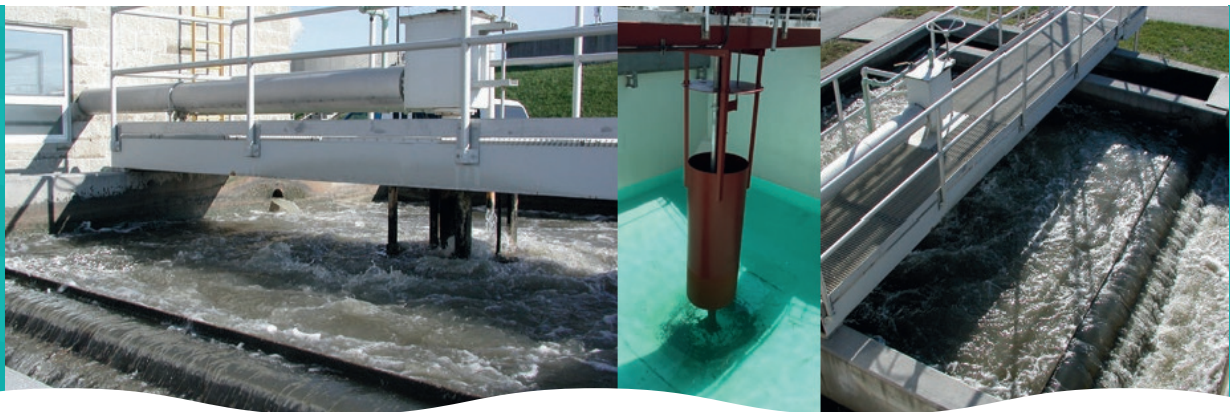
Aeroductor Grit Removal System
