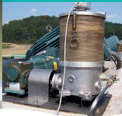
Reservoir with Low Level Switch
